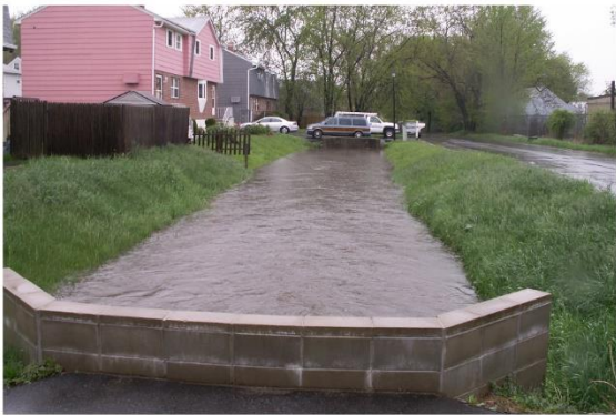
City of Methuen – Bloody Brook Culvert Improvements Bloody Brook at Bicknell Avenue Looking South
